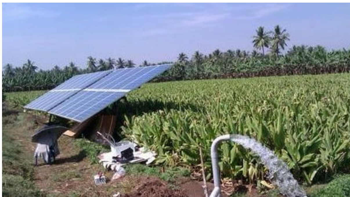
A solar-powered irrigation system
